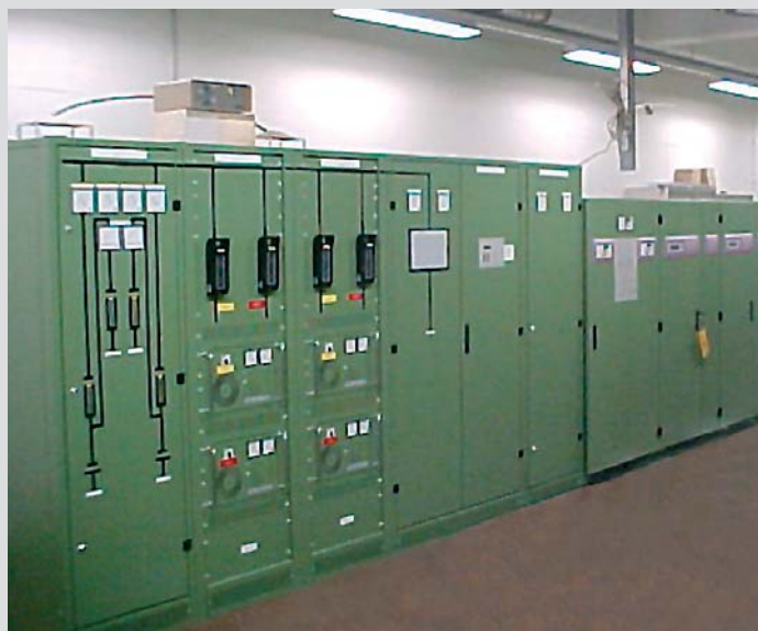
24 V DC supply and 230 V AC UPS unit in power station technology to maintain operation of safety technology at a gas storage facility.
