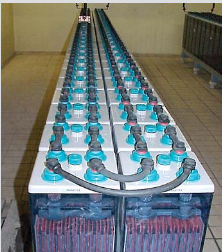
220 V battery unit with a nominal capacity of 1000 Ah to secure the control systems of a power supplier.
